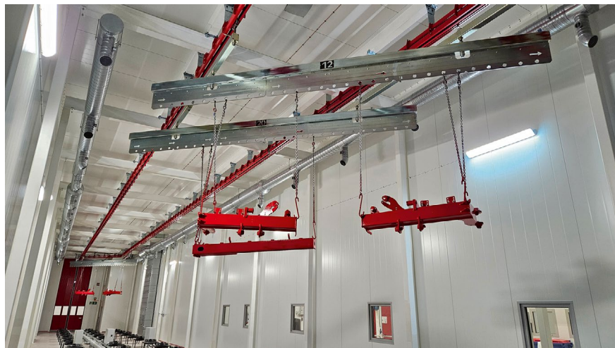
Cross-stacking in a cooling zone.
